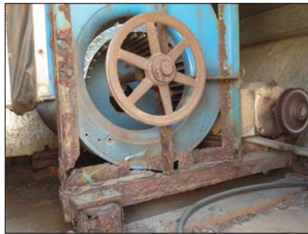
Broken exhaust fan with the motor still running.
