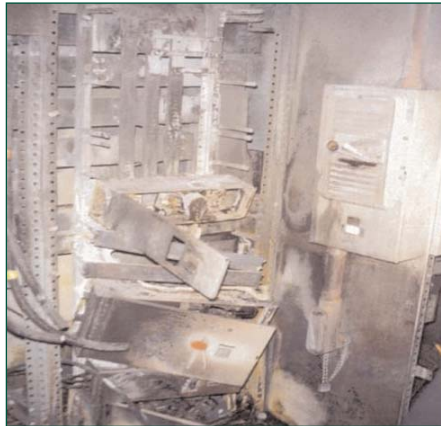
The aftermath of an electrical arc flash
